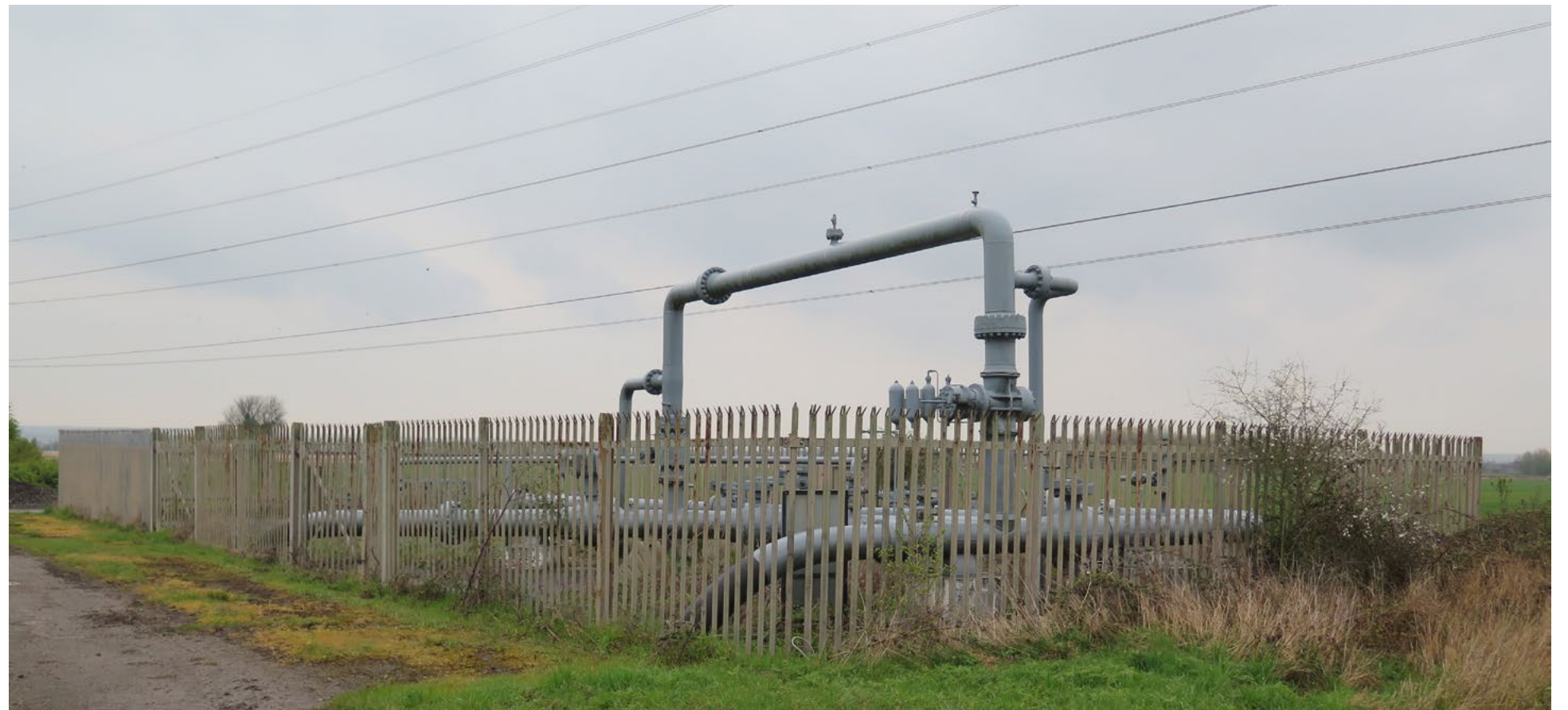
Existing gas compound along FP136
