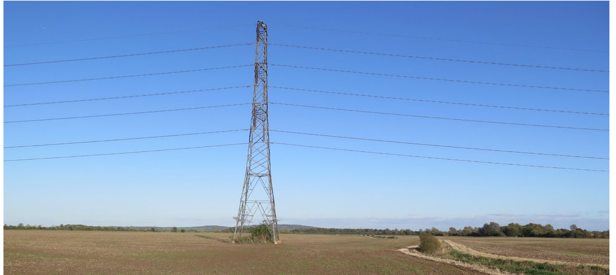
Existing electricity transmission infrastructure looking across Orsett Fen from the Mardyke river
